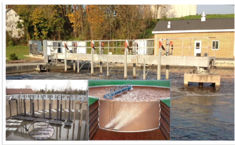
Continuous Flow Sequencing Reactor (CSR) Basin with Moving Bridge, Submerged Diffusers, and Stationary Diffusers
