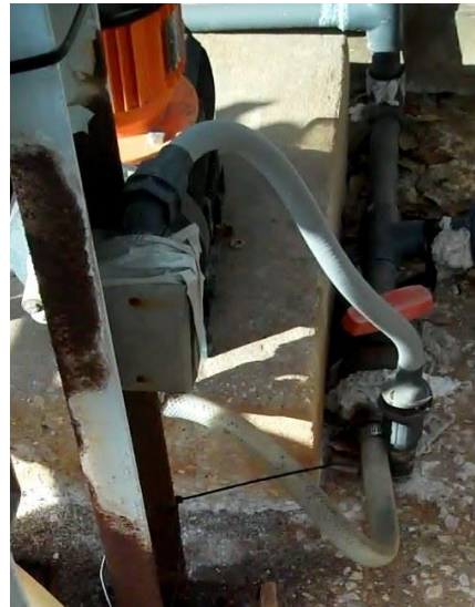
Sealtite Connector Failure
