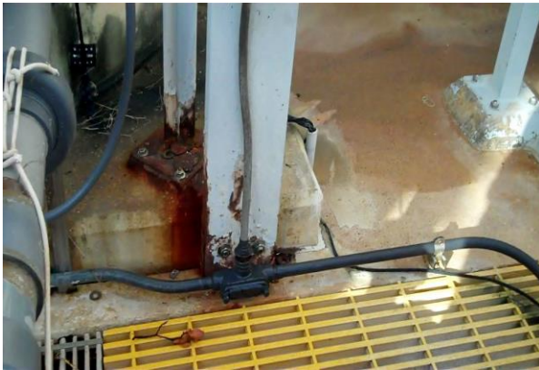
Sealtite Connector Failure
