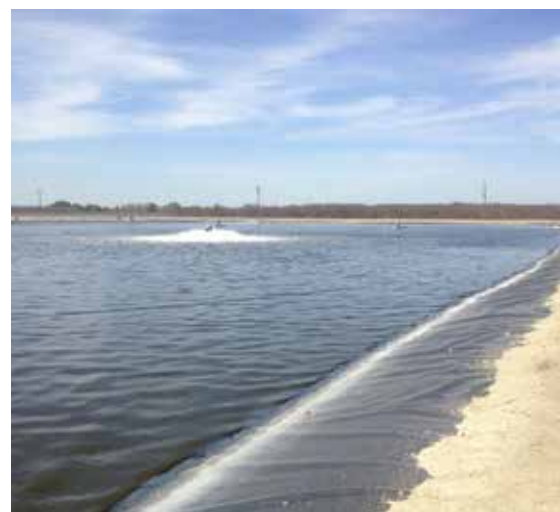
Figure 4: Surface Aerator (in operation)
