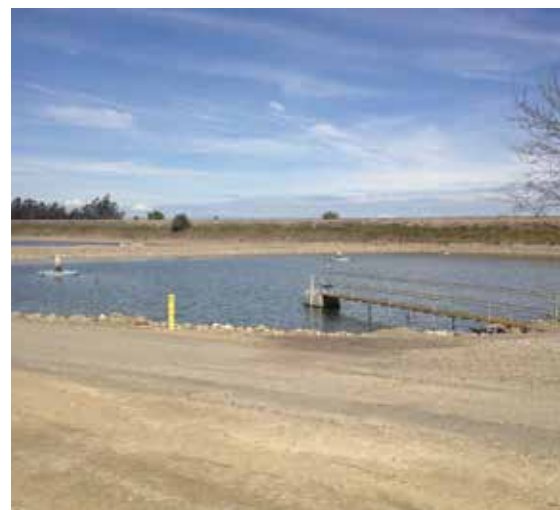
Figure 3: Surface Aerator (idle)
