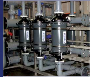
14-inch Industrial system
