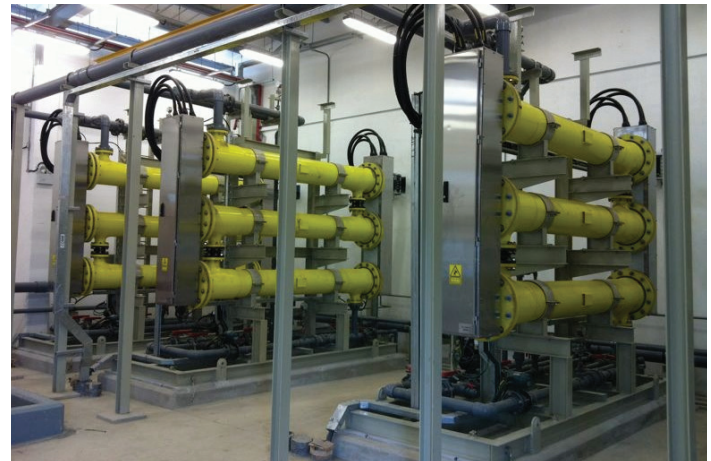
SEACLOR® installation in Keppel Merlimau Cogen power plant, Singapore
