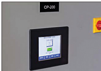
Control Panel Interface
