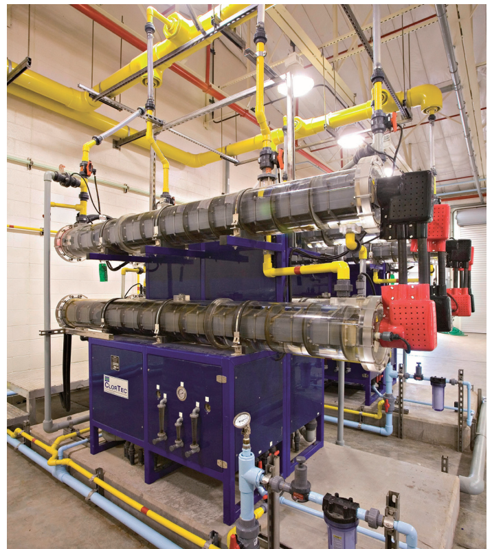
ClorTec CT System at Chandler WTP
