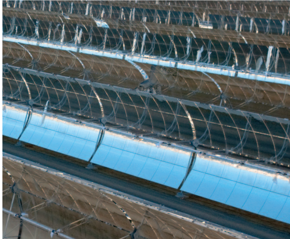
A parabolic trough power plant
