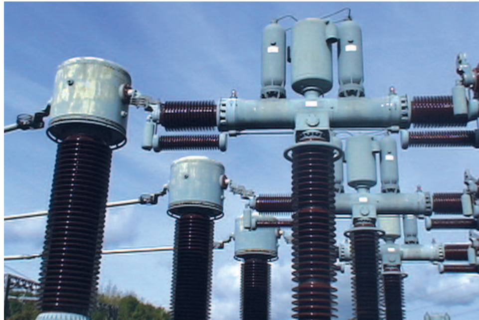
High voltage switchgear
