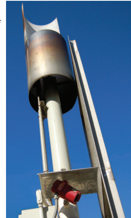
Sierra Steel-Mass™ 640S inserted into landfill flare
