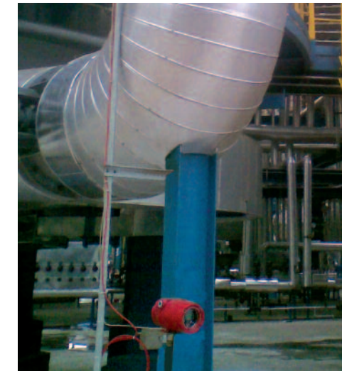
Sierra meter measuring combustion air flow in duct
