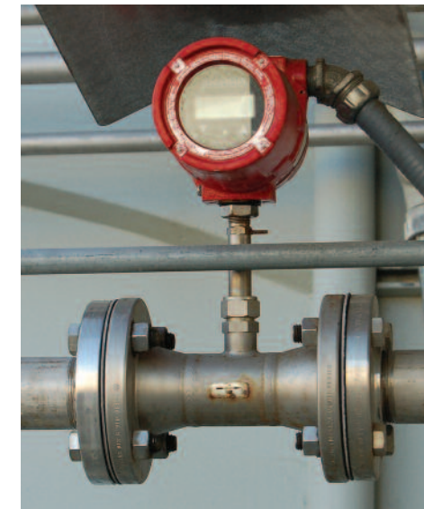
Sierra's Flat-Trak™ 780 at Santa Cruz Wastewater
