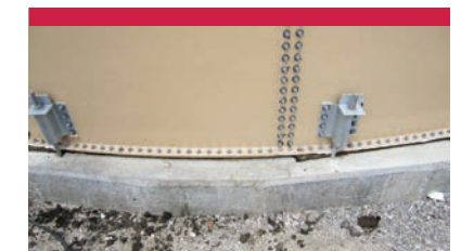
» Anchored to Slab Foundation Tanks are anchored to slab with anchor bolts around perimeter
