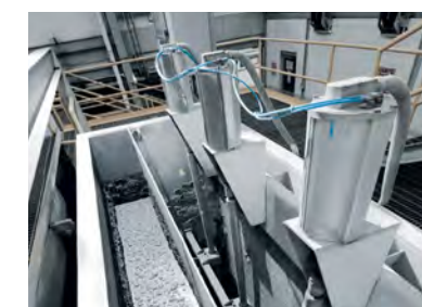
Control of dart valve for level regulation in mineral processing
