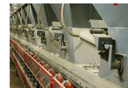
Control of silo discharge in fertilizer processing
