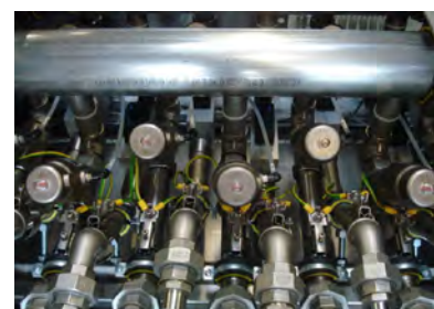
Water cooling systems
