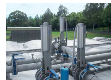
Controlled sluice gate for flowrate of return sludge at a wastewater treatment plant
